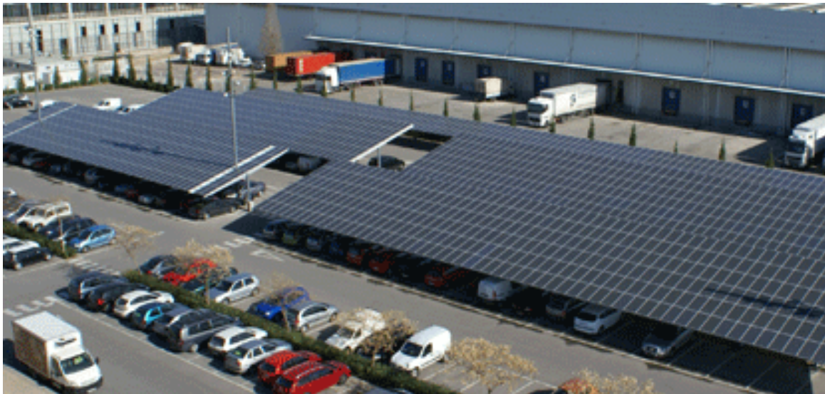
Photovoltaic installation in the port of Barcelona
