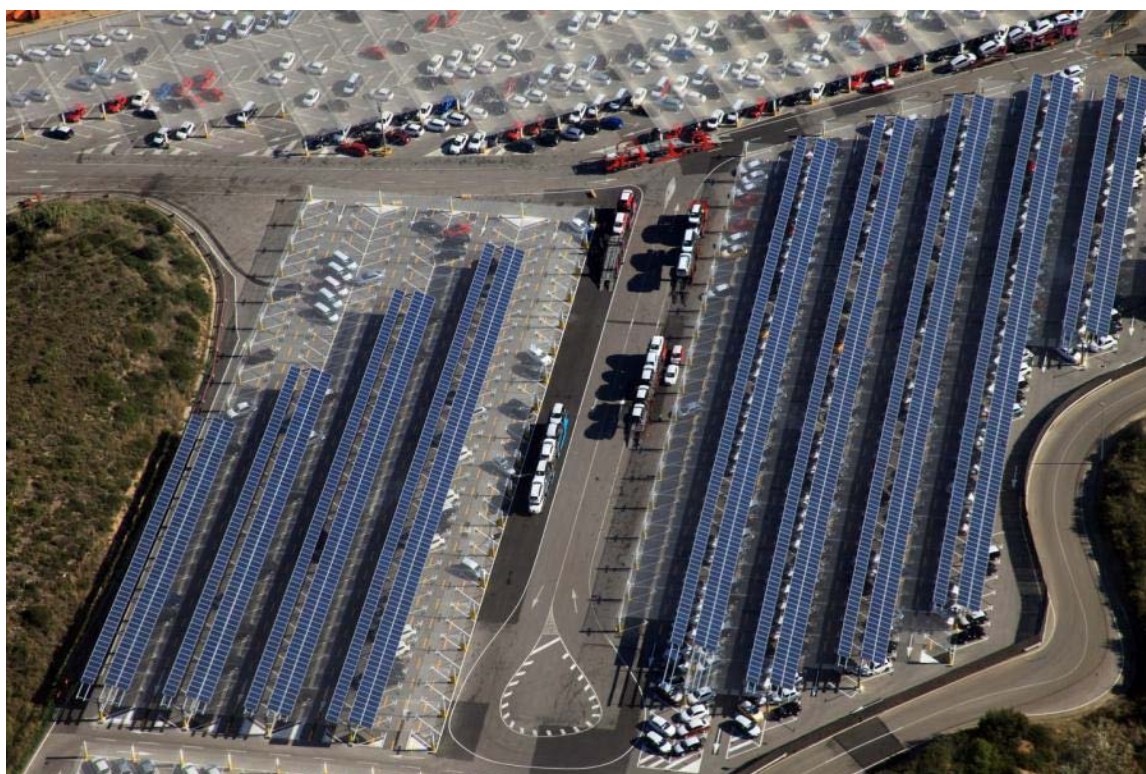
Photovoltaic installation in the SEAT factory
