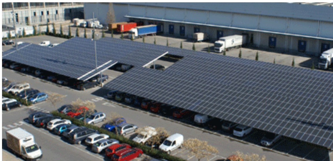
Photovoltaic installation in the port of Barcelona
