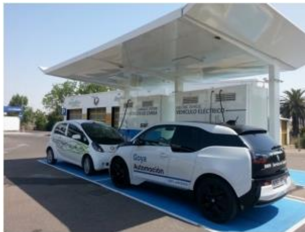
Charging point in Zaragoza. Source: Ecoticias
